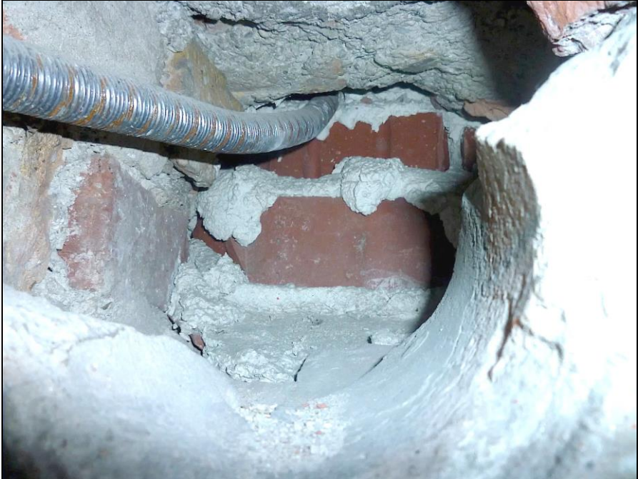
Document 62: Dachau Crematorium, Room 7, remains of the observation opening between Rooms 7 and 8. Source: Rudolf.
