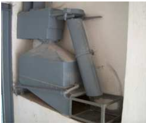
Photo 15: Hot-air fumigation device.
