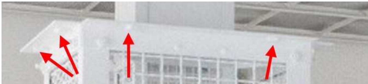
Illustration 7: Anchoring bolts in Kula's column according to van Pelt. Section enlargement of Illustration 3.
