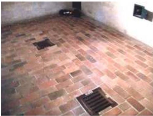
Photo 3: Gas chamber floor.
